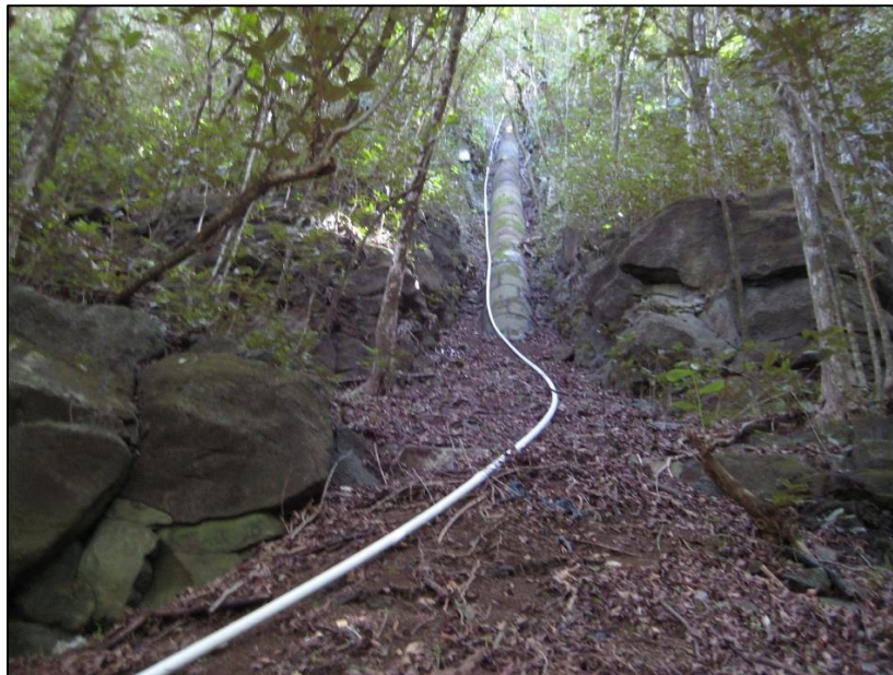
Figure 12. PVC-pipe system in Māliko gulch
